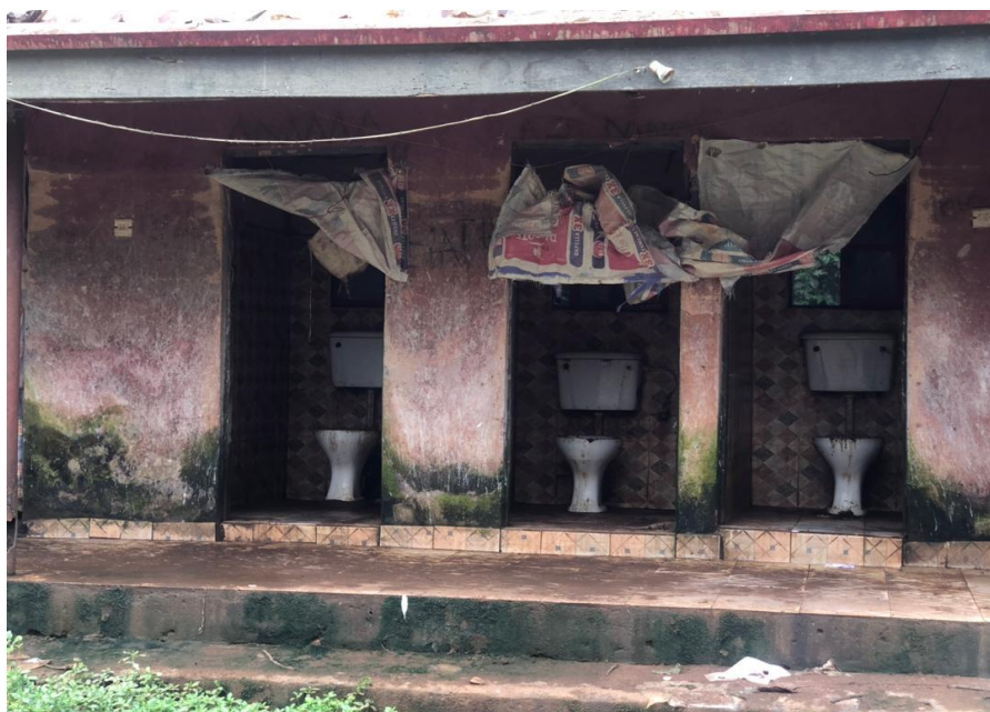
Fig 4: Unclean toilet facilities without doors.
