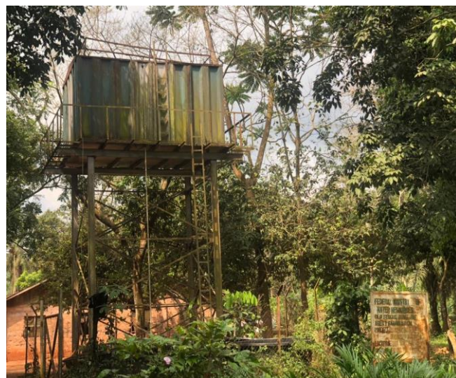
Fig 2: Abandoned solar-powered borehole
